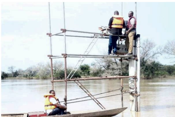
Figure 25: Installation and Rehabilitation of Hydrometric Gauges in Black and White Volta Rivers
